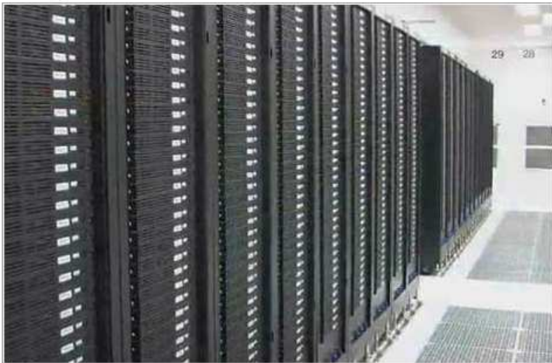
A look at the dense server configurations in one of the 97 data centers operated by Intel Corp, which runs more than 100,00 servers.
